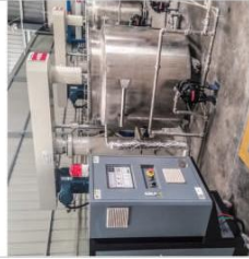
■ The Imperature control of agitator tank
